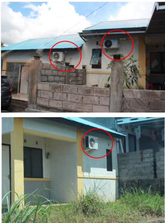
Fig 7_ Air conditioning is essential for ensuring the optimal thermal comfort of the house's occupants
